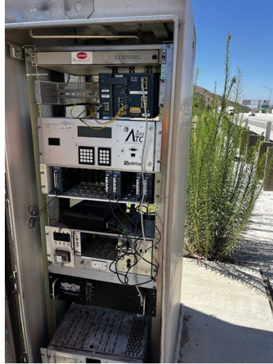
Figure 3: No power at previously deployed SR-57 @ Diamond Bar TAMS site
