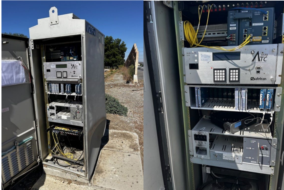
(a) Damaged cabinet at SR-60 @ Bixby (b) Relocated setup at SR-60 @ Albatross
