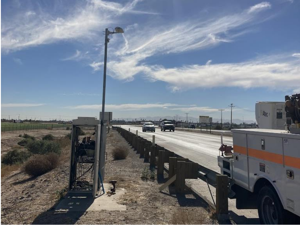
Figure 2-4 Equipment Setup at SR-7 Calexico
