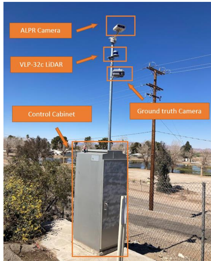
Figure 2-2 Example of Sensor Installation at Blythe Study Site
